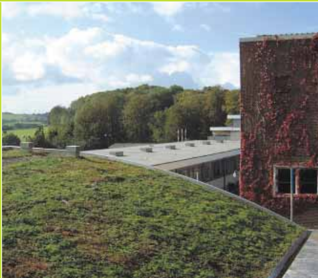
House for the Future, Museum of Welsh Life, St Fagans. Sedum mat installation
