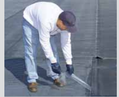
Clear poly backing is removed from the Factory-Applied Tape before seams are rolled
